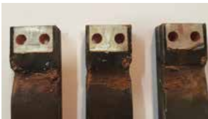
Fig. 1: Arc fault damage
